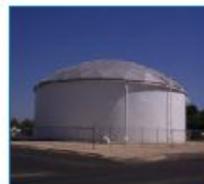
Field Erected Tanks
